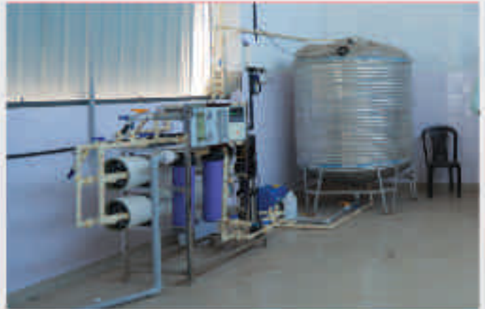
RO/UV water purifying plant
